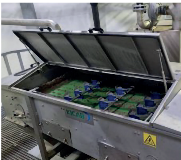
Sludge processing unit at Kjærelva.
