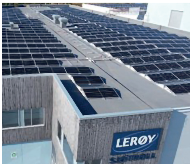
Solar panels at Kjærelva.
